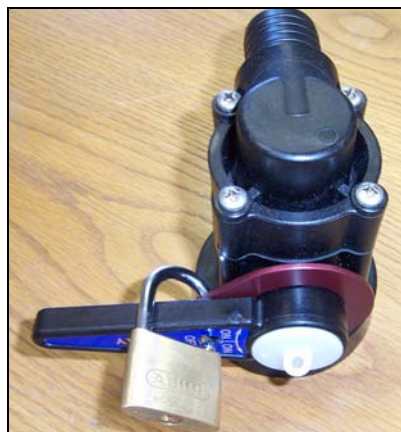
Valve closed and locked
